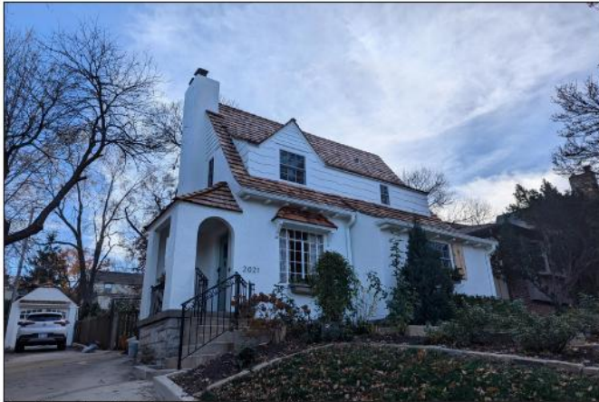
1. Primary (north) and east elevations, View SW Part 2 Scope Item #1: exterior painting
